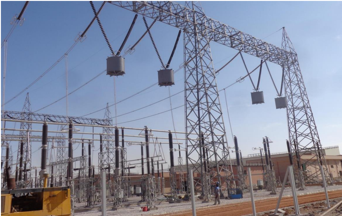
Figure 1; A 420 kV Air Insulation Substation, Middle East, 2018
