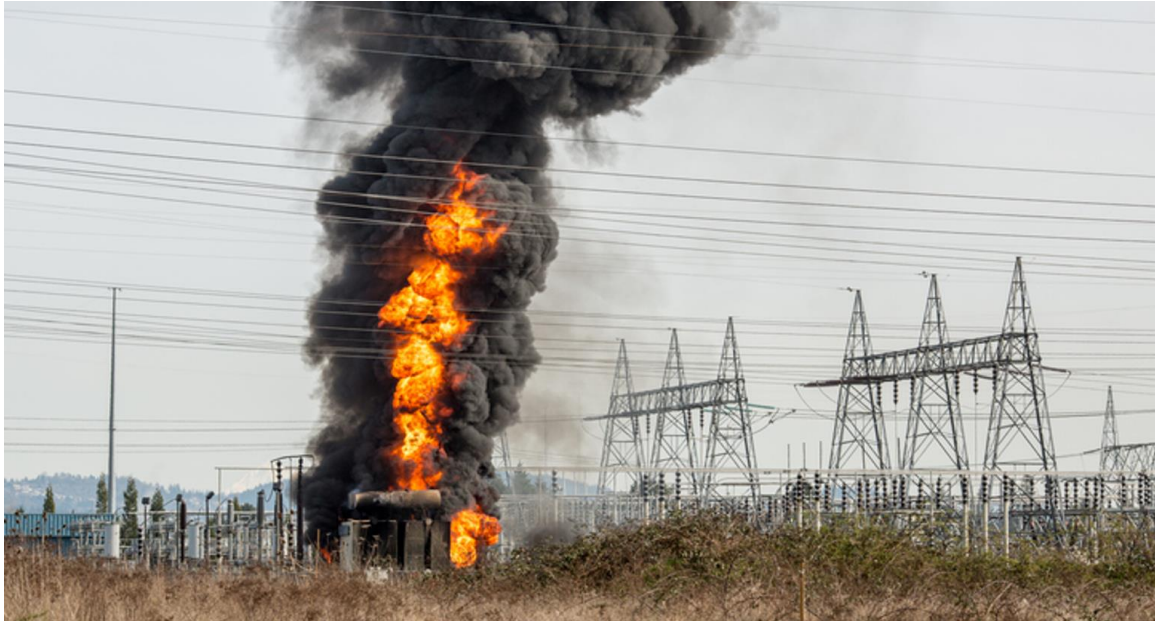
Figure 4; A 69 kV oil power transformer caught fire,
