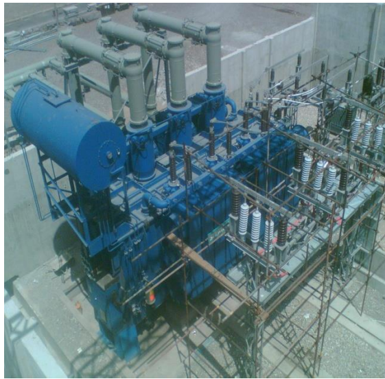
a) Step-up Transformer
